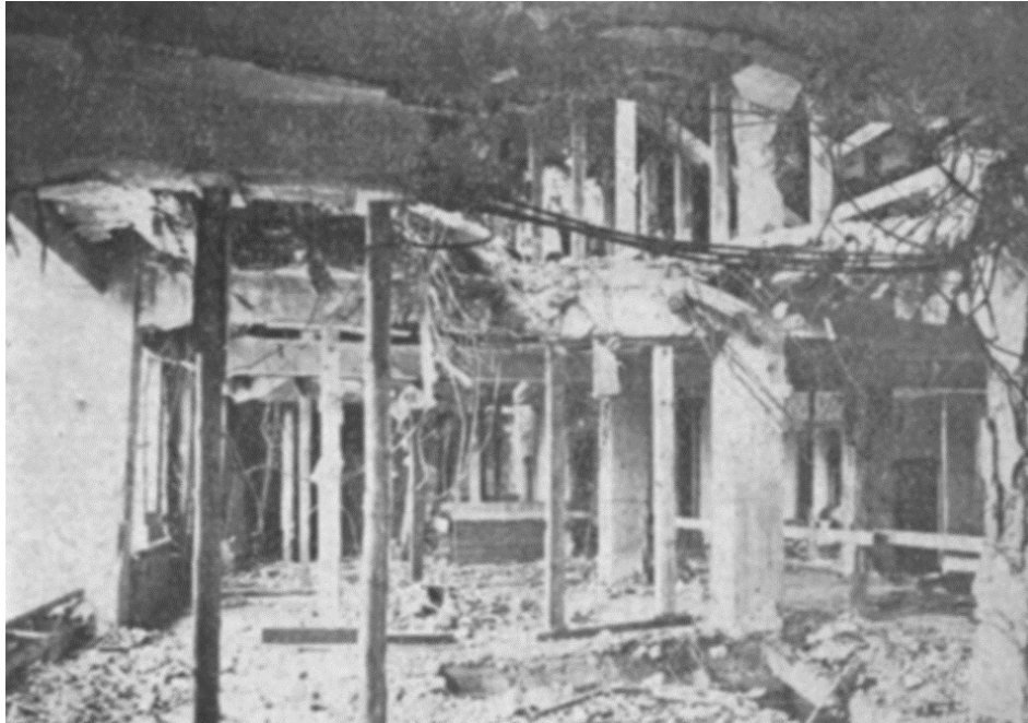
Fig. 4. Damage caused by the German bombing in September 1939. An entire span and part of the floor is missing [4]
